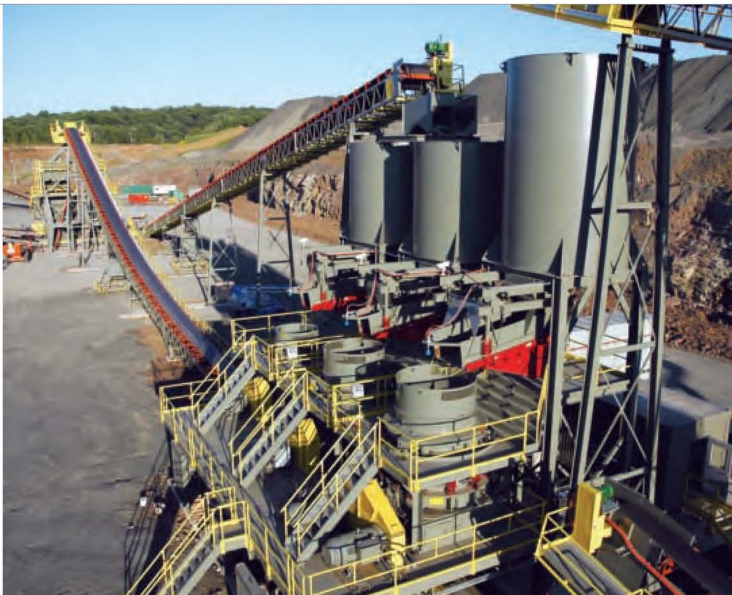
Automated 1000 TPH crushing plant with 68SBS, 57SBS and 52SBS cone crushers
